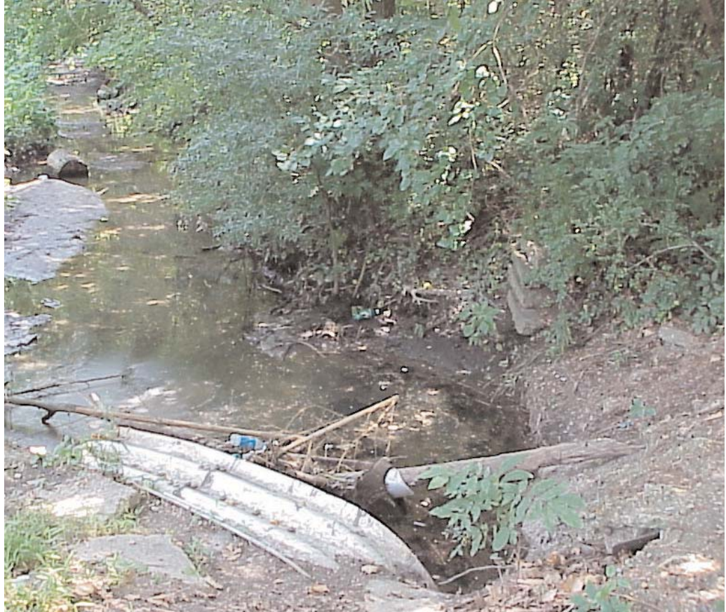
This degraded ditch in the Lenox neighborhood is being transformed into a large stormwater wetland.
