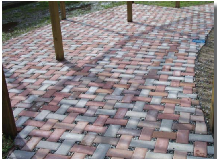
Norfolk Environmental Commission used volunteers to install this attractive pattern of bricks for its permeable, or rain-absorbing, sidewalks around the Ernie Morgan Environmental Action Center.
