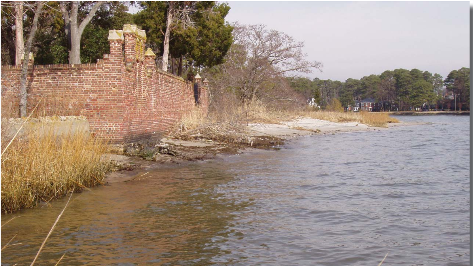
Before- A wetland at the Hermitage Museum in Norfolk, VA was eroding, threatening the historic wall and providing severely degraded habitat.
