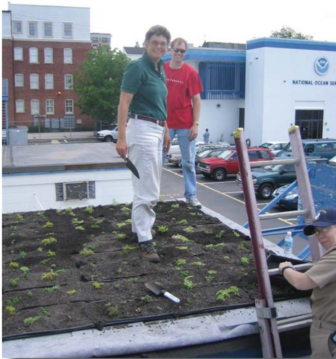
Succulent plants and engineered soils now filter runoff and extend the life of roofs on several of its smaller buildings at NOAA Marine Operations Center Atlantic in Norfolk, VA. Here, Pam Boatwright, River Stars program manager, and Doug Smith, NOAA work with volunteers on installation day.
