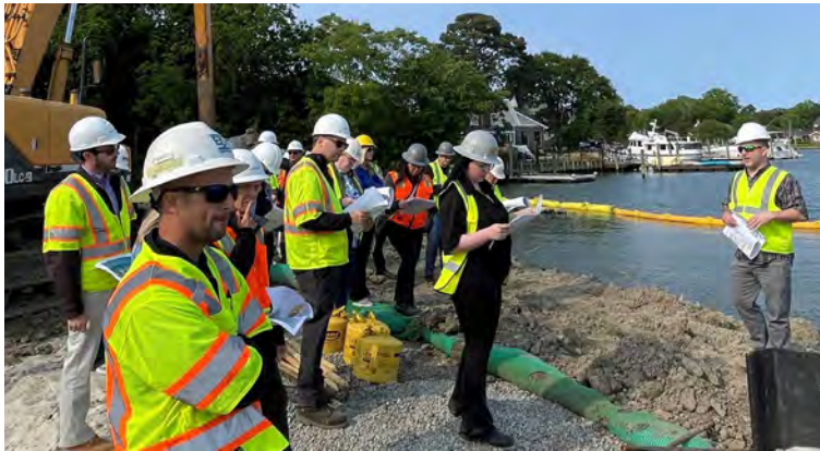
The Ryan Lab drew the best turnout of any recent hard hat tour of the American Institute of Architects, Hampton Roads Chapter. Mike Fox, Stromberg/Garrigan & Associates (R), explains the “living shoreline” underway, replacing a failing marina.
